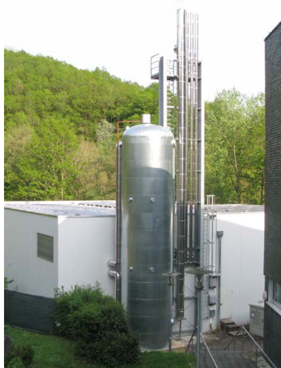
Fig. 06-8 Central heat store
