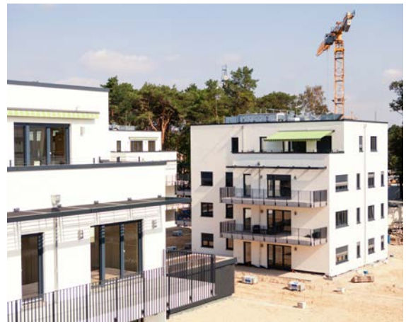
Heat transfer/house connection
