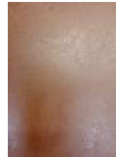
11_IR_RT * IRON RUST
