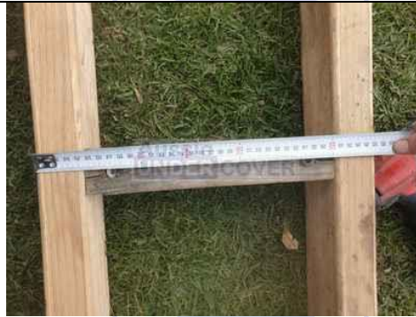
Outside to outside 350mm wide 90 x 45 treated pine. 20mm form ply will be added to each outside edge.
