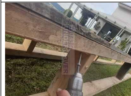
Screws must be accessible once the concrete has been poured so the form work can be removed
