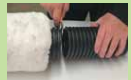
Cut pipe – ensure you leave enough pipe so it will accommodate joiner
