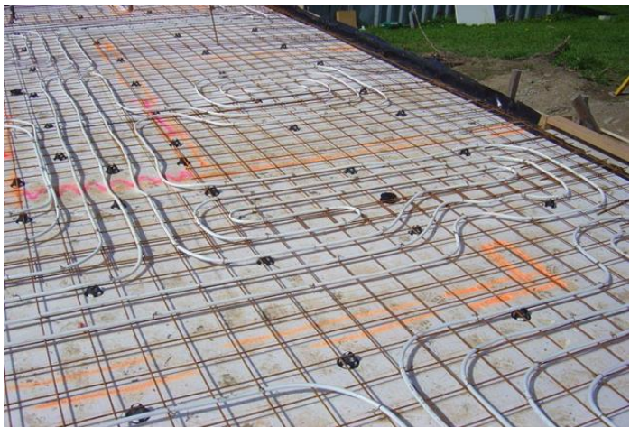
Underfloor Heating Pipes attached to reinforcing mesh. Walls marked out in day-glow paint on polystyrene
