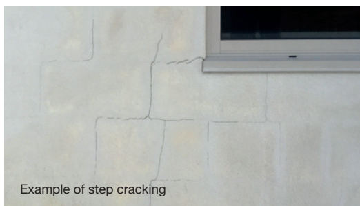
Major cracking such as in this example should be assessed by a building professional
