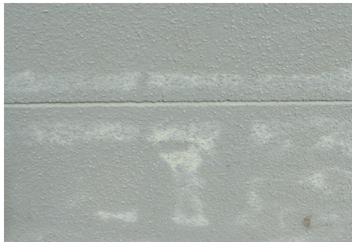
Example of Efflorescence
